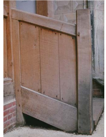
Figure 9.1.9 Timber in the splash zone darkened rapidly Photo: P Ross
