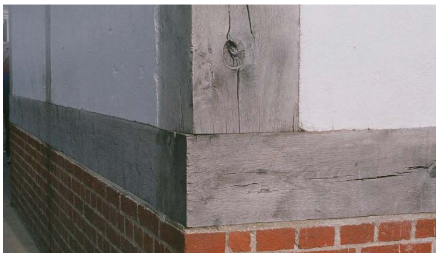
Figure 9.1.6 Slight twist at the base of one of the posts in the north-east tower Photo: P Ross
