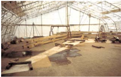
Figure 9.5.6 The temporary covered workshop set up on the north side of the nave. The plywood floor is painted white and the truss profiles drawn on it. In the photograph, two trusses have been fabricated and stacked to one side by lifting with shear legs Photo: P Ross
