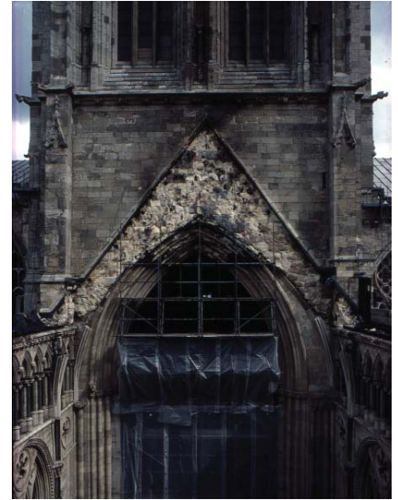
Figure 9.5.2 The south face of the central tower immediately after the fire, showing the dripstone which sets the line of the roof, and below it, the line of the vault Photo: P Ross
