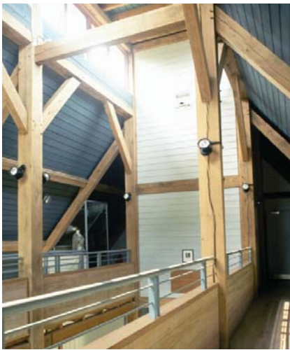
Figure 9.6.1 Bedales School Theatre from top: Exterior Photo: P Ross Foyer gallery access Photo: P Ross
