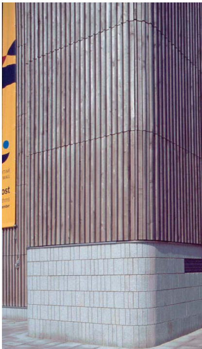
Figure 9.9.4 Alternate batten detail used on the curved wall surrounding the main entrance Photo: P Ross
