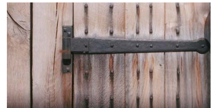
Figure 9.1.10 Staining from the iron nails in the door Photo: P Ross
