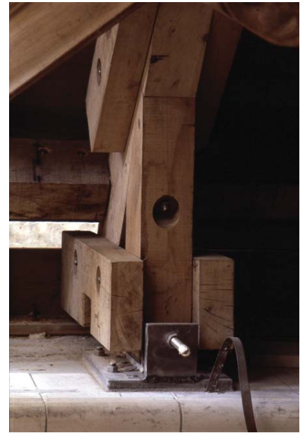
Figure 9.5.8 The east truss legs rested on a sliding bearing and were restrained by a threaded rod engaging with the upstand arm of a cleat bolted to the masonry. As the load of the roof boards and lead covering were applied, the leg restraint was gradually released by unscrewing the nuts in sequence, a quarter-turn at a time. Most of the out-thrust was dissipated, leaving the scissors acting as true trusses Photo: P Ross
