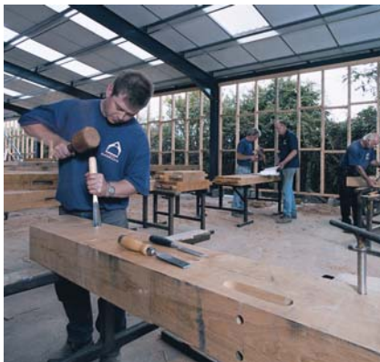
Figure 6.5 After main preparation using Hundegger equipment, green oak framing work is completed using traditional hand tools Photo: T J Crump Oakwrights
