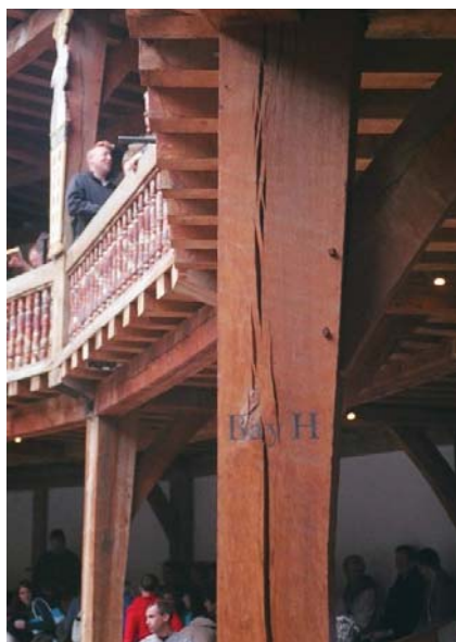
Figure 9.1.4 The major fissure in one of the ground floor posts Photo: P Ross
