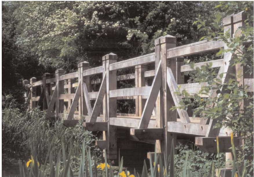
Figure 8.21 Green oak bridge at Whitchurch, Hampshire with triangulated parapet supports Photo: The Green Oak Carpentry Company Ltd
