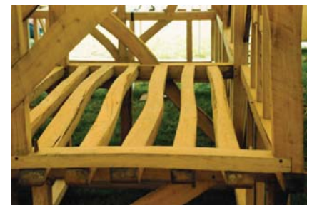
Figure 6.11 Floor joists, traditionally hand sawn only on what became the upper and lower faces, placed “flatwise,” and hence providing a level floor
