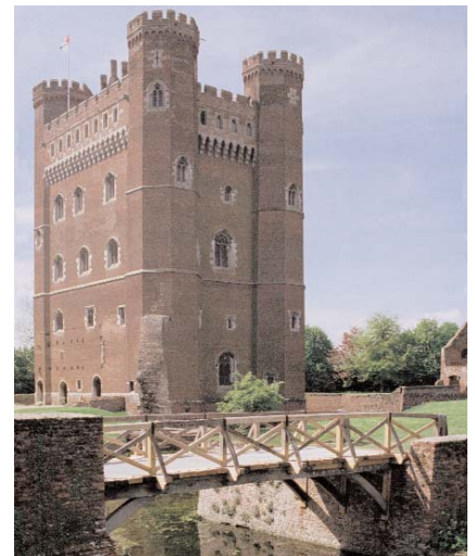
Figure 8.18 The Moat Bridge, Tattershall Castle, Lincolnshire. An English oak structure recently repaired, typical of the many small bridges crossed by large numbers of visitors to properties in care Photo: Wood Awards
