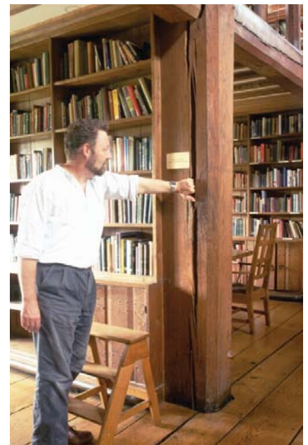
Figure 5.7 Significant fissure in a post in Bedales School library, built in 1921 Photo: P Ross
