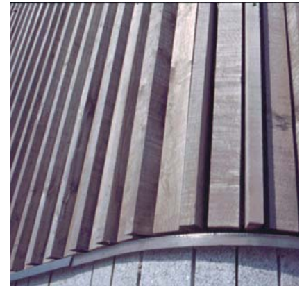
Figure 9.9.7 Detail - metal drip protecting the masonry below from tannin run-off Photo: P Ross
