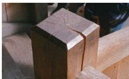
Figure 9.1.5 A newel post with boxed heart showing radial fissures. The handrails, being quarter-sawn and excluding the heart, have few fissures. The polish on the top of the post is entirely due to hand contact Photo: P Ross
