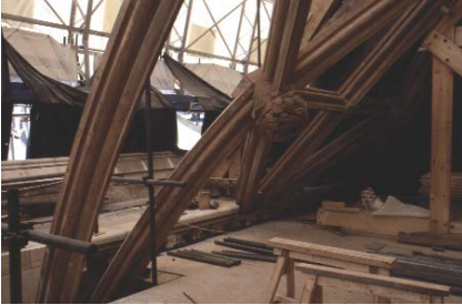
Figure 9.5.11 The assembly of the vault, with ribs tenoned into bosses (also made from oak strips, brick bonded to keep the grain in one direction out of consideration for the carvers)
