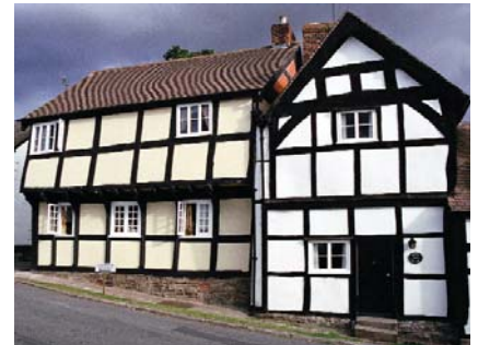
Figure 8.2 The technique of building oak frames using sill beams mounted on stone or brick was developed quite early, because earth-fast posts rotted quickly. A horizontal sill beam resting on a low stone wall resists ground water because moisture absorption across the grain is much more limited than through the end grain. In conjunction with modern damp proof courses and flashings, this is still best practice (Weobley, Hereford and Worcester)
