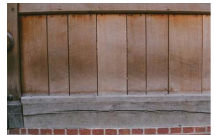
Figure 9.1.11 The sill beam, showing water marking and darkening on the planking above where 'groundlings' squat on the beam Photo: P Ross
