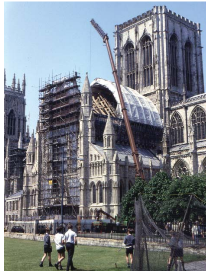
Figure 9.5.7 Lifting four complete trusses in one day required a crane with a lifting capacity of four tonnes at a twenty metre radius, but this was an economic alternative to dismantling and re-erection Photo: P Ross
