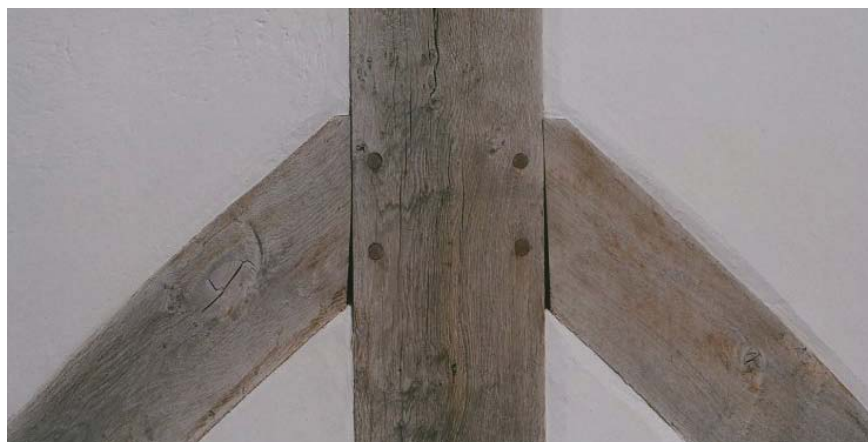
Figure 9.1.7 The typical wedge-shaped drying movement at the ends of the wind braces Photo: P Ross
